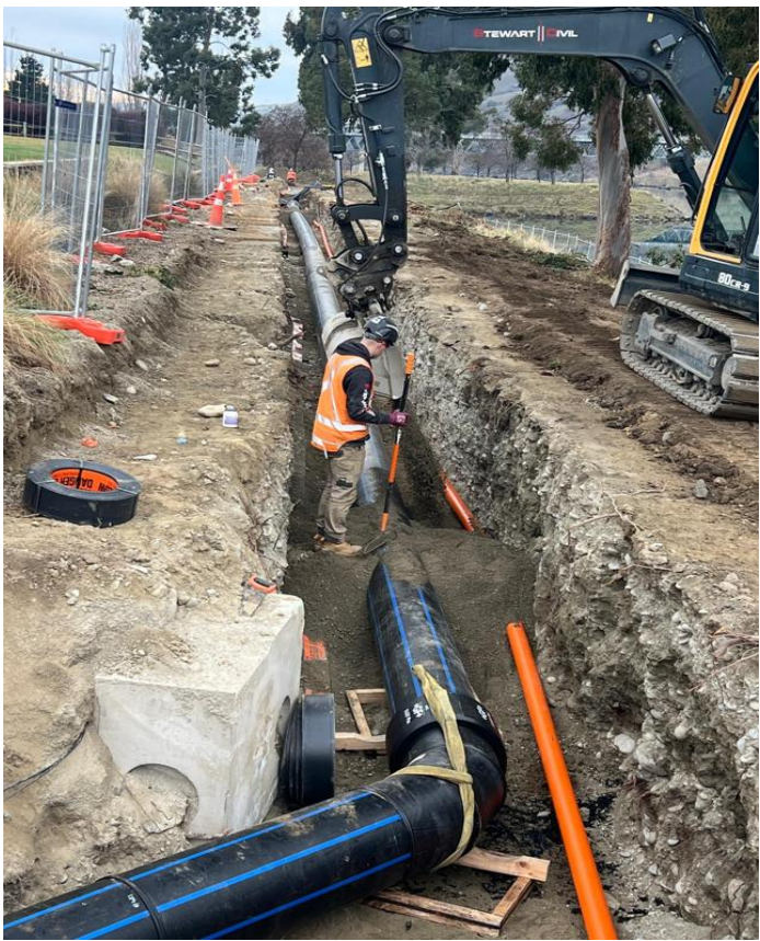
Above: Pipework from borefield to rising main
