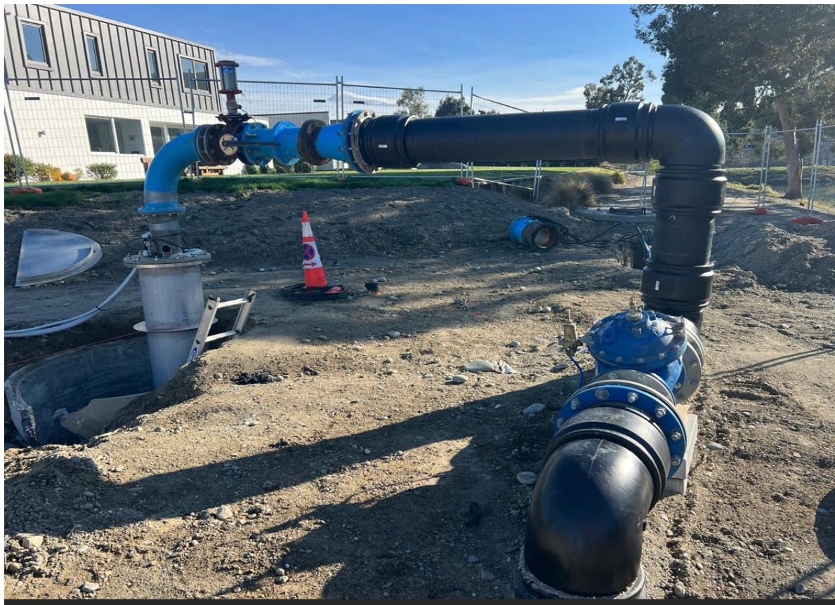
Above: Borehead pipeworks adjacent to Alpha Street reserve
