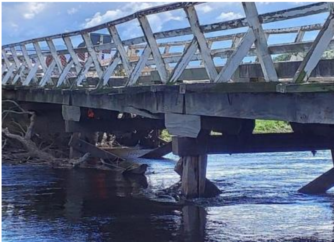
Maniototo Road bridge damage
