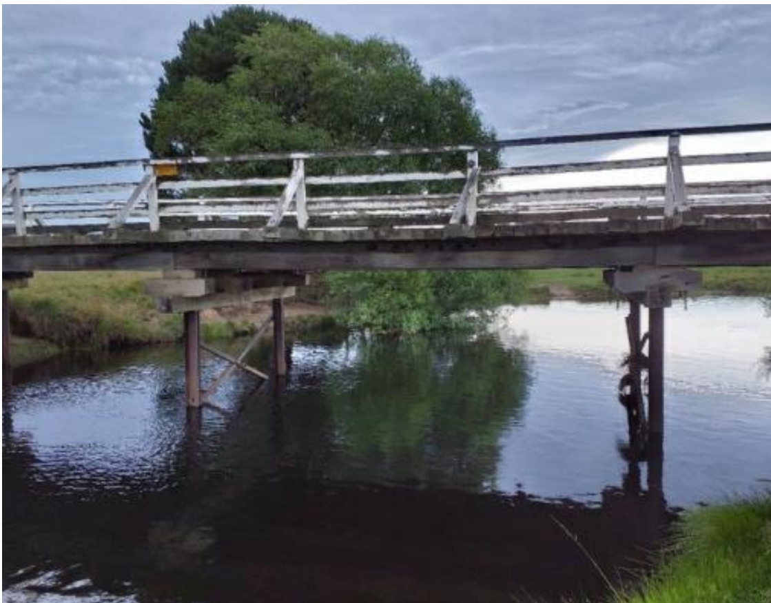
Linnburn Runs Road bridge damage
